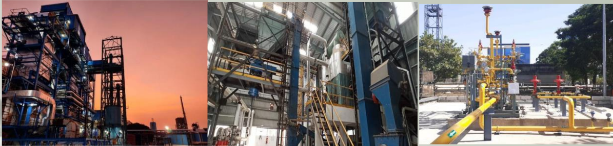
(L to R) Cogeneration power plant; Biomass briquette boiler; Direct high-pressure gas system
