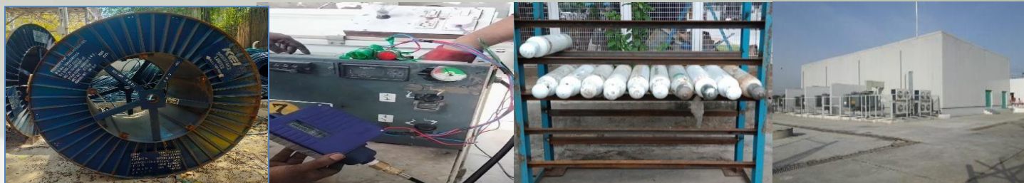
(L to R) Cable drum recycling initiative; S6 Manometer; SF6 cylinders and Battery Energy Storage System (BESS)
