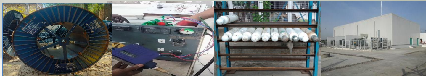
(L to R) Cable drum recycling initiative; S6 Manometer; SF6 cylinders and Battery Energy Storage System (BESS)
